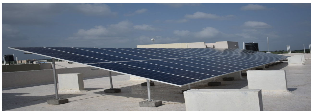
SOLAR PV PLANT AT THE COLLEGE AND SARASWATI GIRLS HOSTEL HOSTEL FACILITIES
