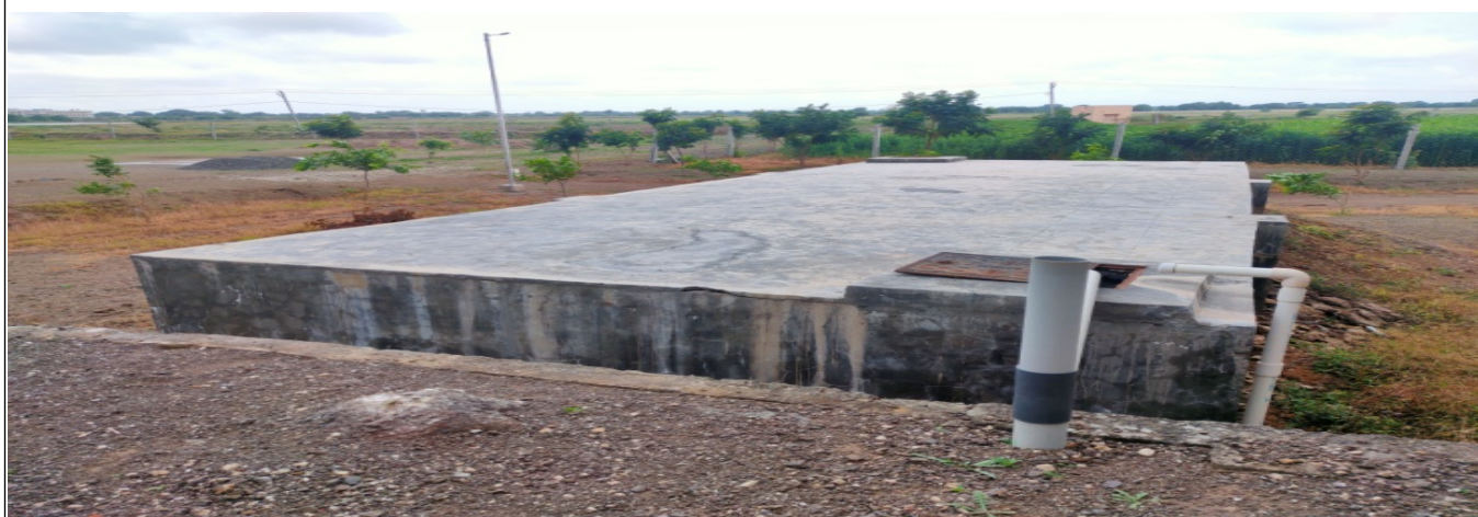
WATER HARVESTING TANK
