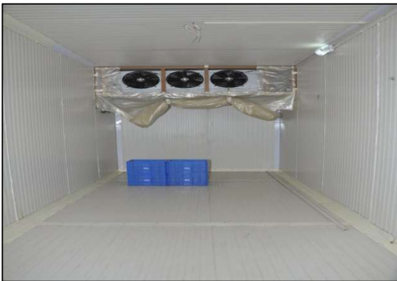
PRE COOLING CHAMBER
