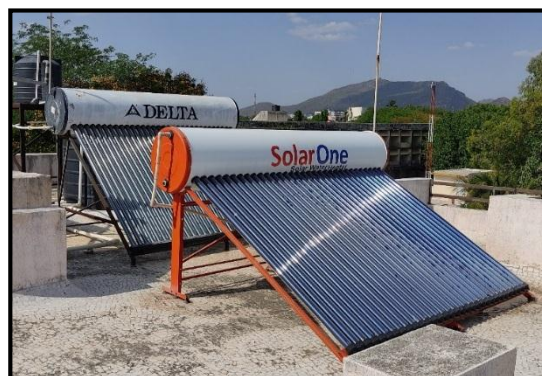
Solar Water heater
